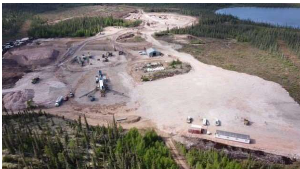
Figure 2 - Overhead image of site with ore sorter in the foreground and pit in the background
