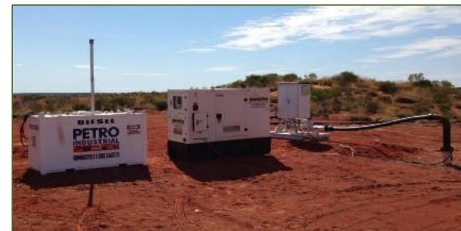
Typical Bore Pump Station
