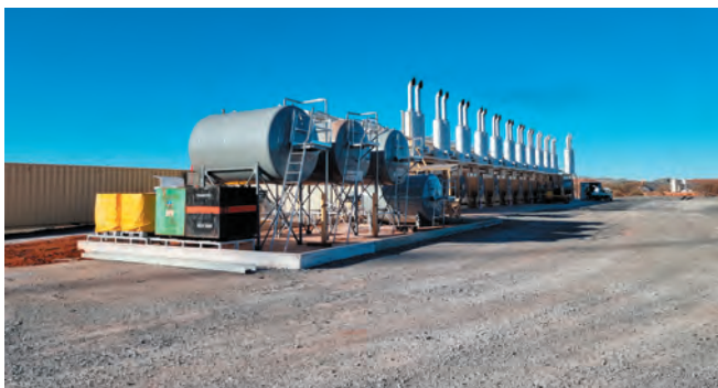
New temporary power station
