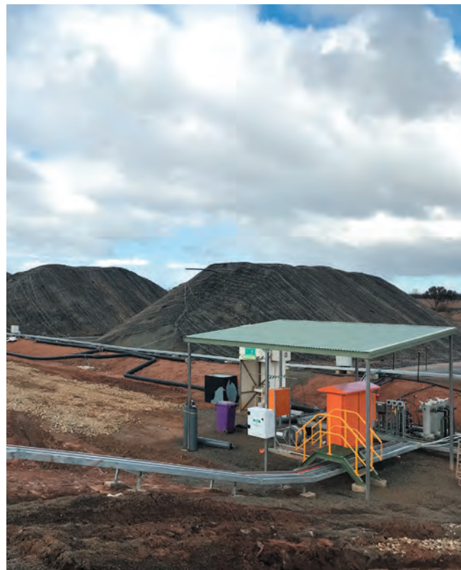
Scats Heap Leach - Heaps in the background with pump station in the foreground. PLS collection facility on the RHS.
