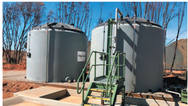
Scats Heap Leach – Acid storage tanks.
