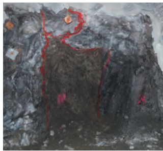
385 S1 south ore drive (4.0m W x 4.5m H) with a face grade of 3.2% Ni
