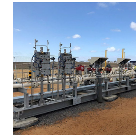
AGIG / Mitsui E&P Scope: Deliver the Waitsia Metering & Offtake station. SMP - Xyris gas plant & compression upgrade project
