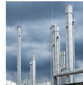
BMT Scope: Fabrication of vessels, tanks, piping and structural steel - Mercury Waste Treatment Facility in Kwinana
