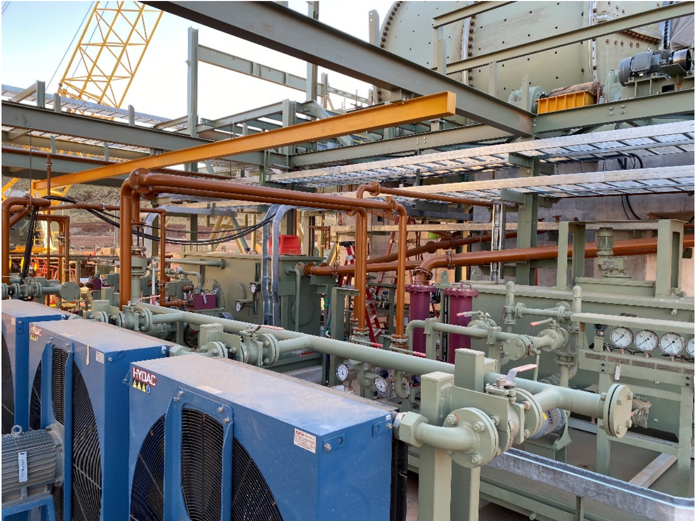
Figure 3: Mill Lubrication System installed
