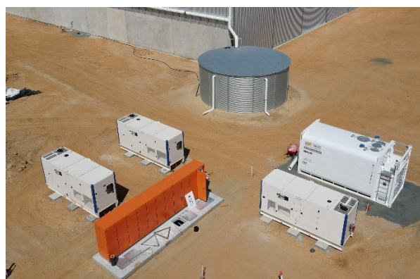
Figure 4. Gensets installed on-site at the Wickepin Project
