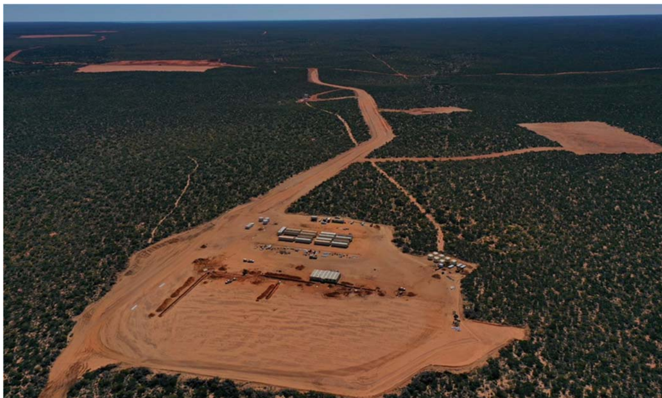
Figure 2 Widespread Construction is Advancing at Strandline's 100%-owned Coburn Project in Shark Bay, WA
