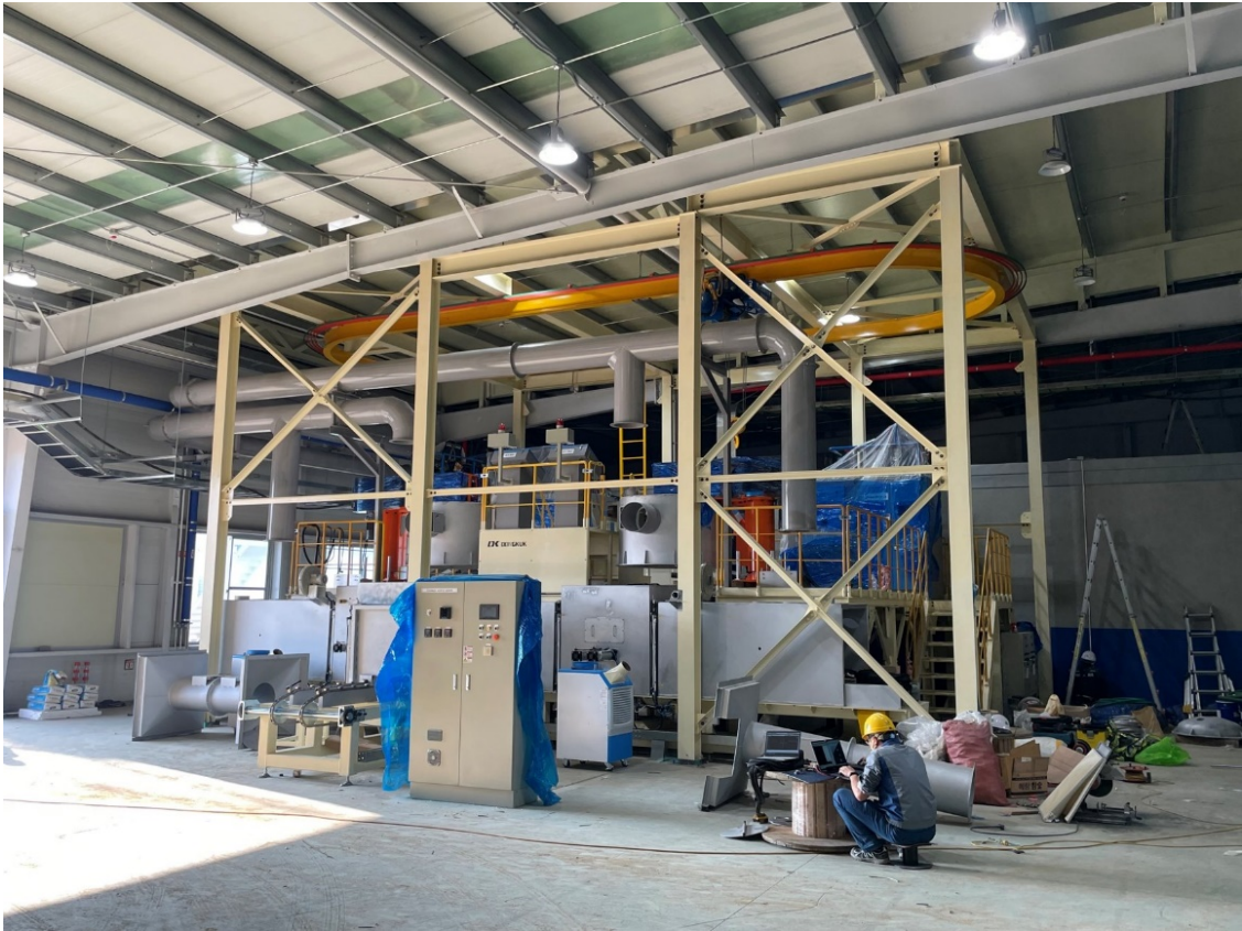
Figure 2 - First two Titanium Furnaces Installed
