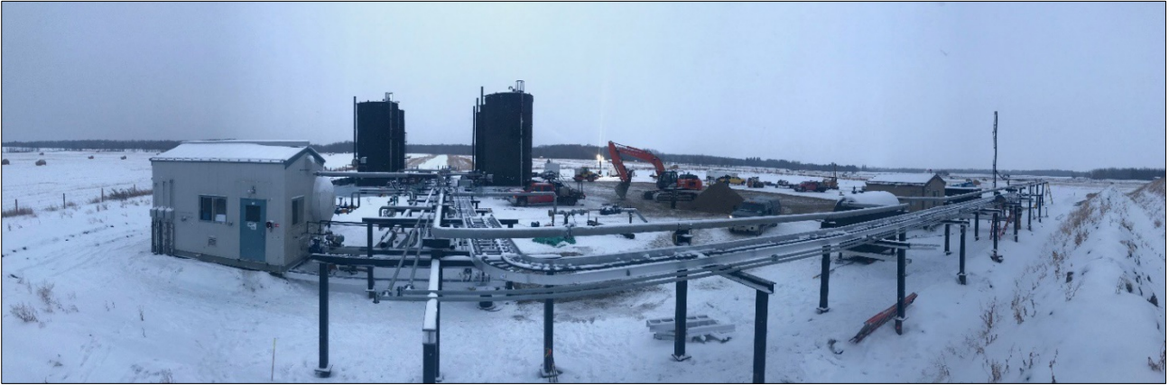
Figure 4 - Installed and commissioned upgraded Wizard Lake Facilities
