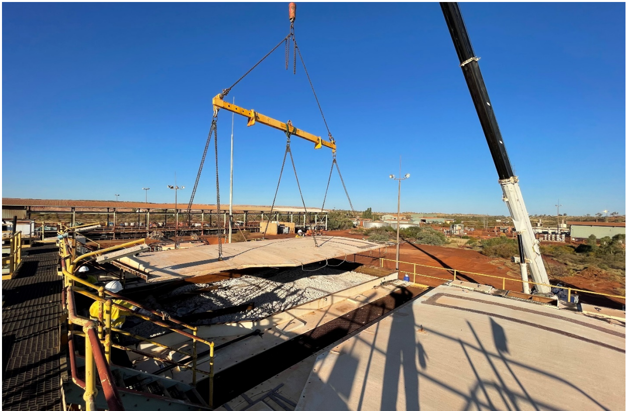
Image 10 | Settler Lid removal at the Solvent Extraction Plant
