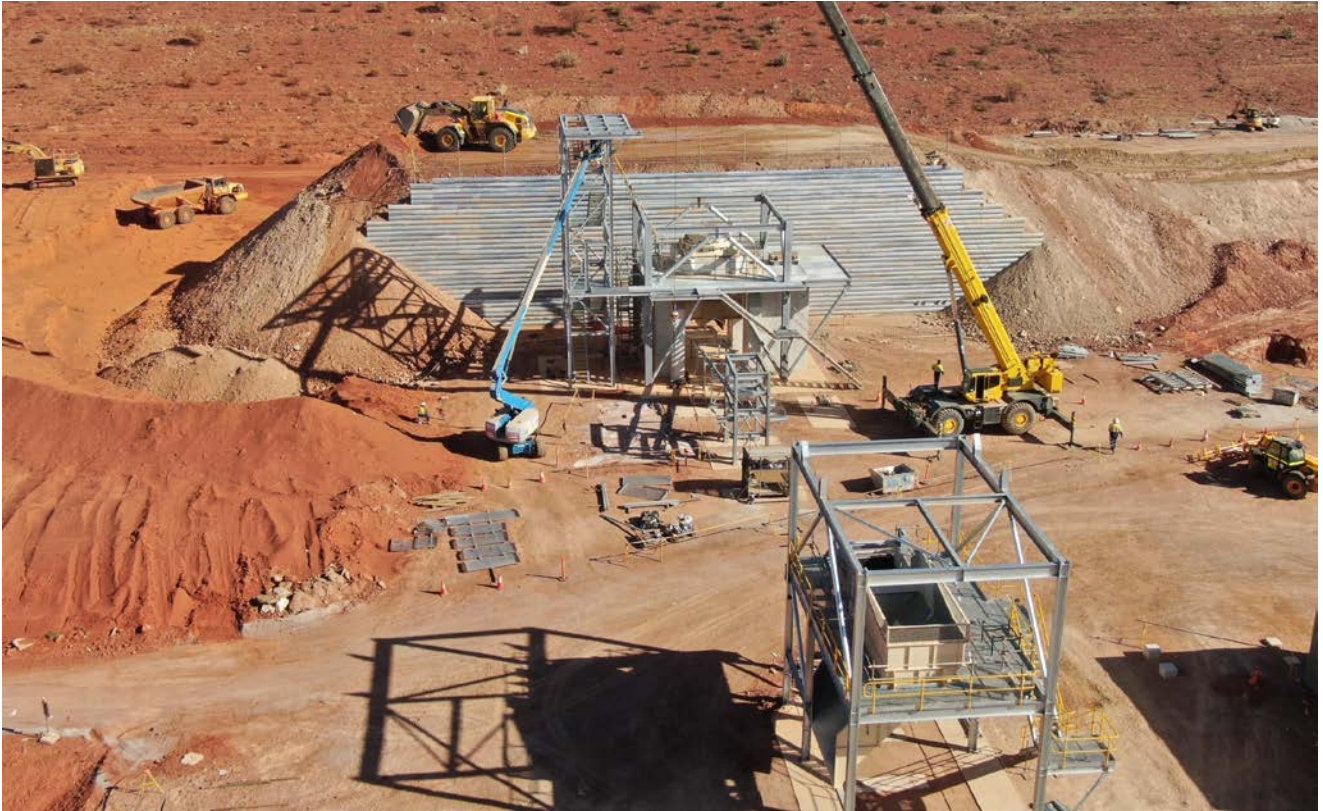
Figure 2: Gyratory crusher base installed, the main frame assembled, and structure being erected.
