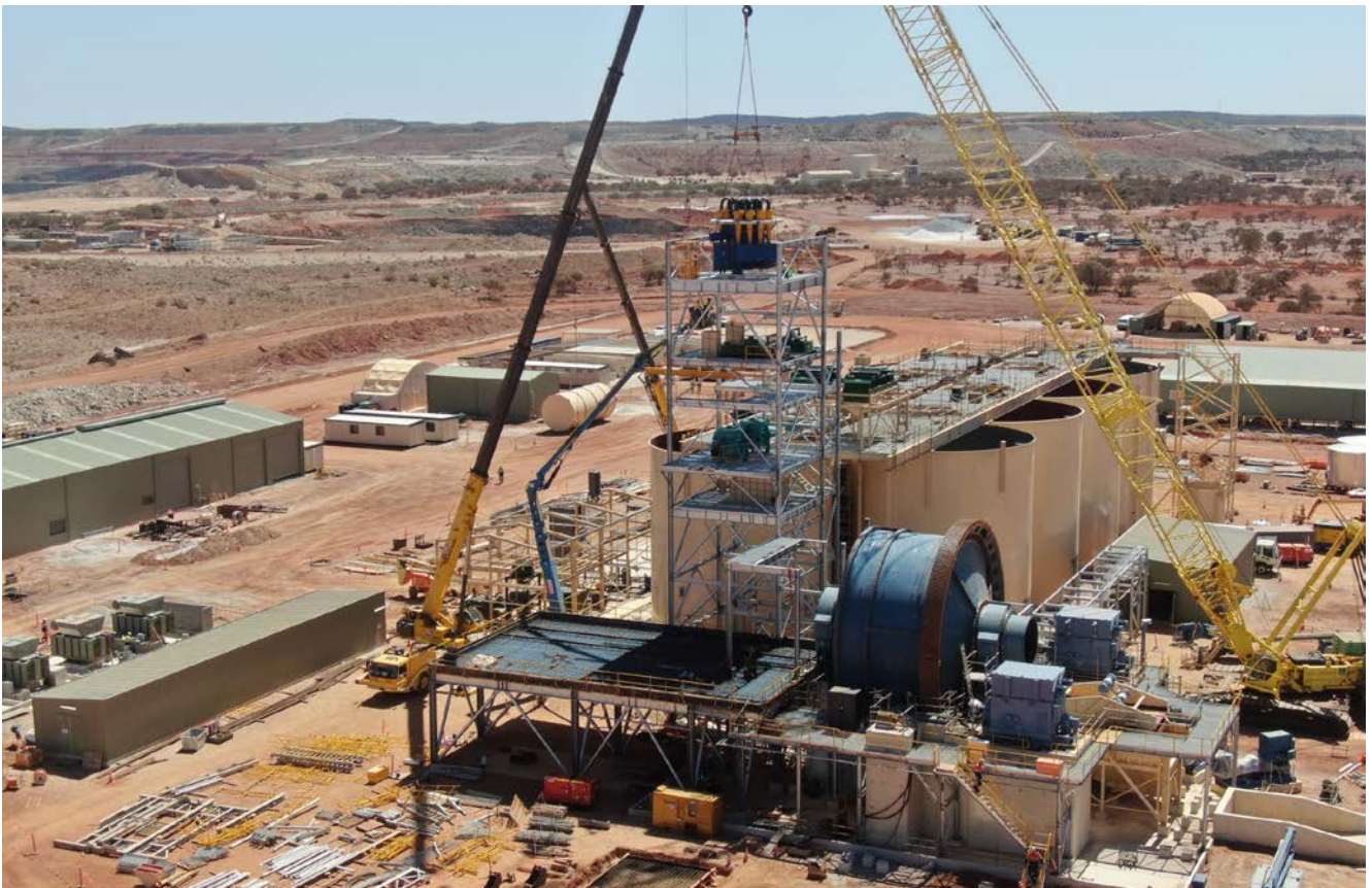
Figure 3: Cyclone being lifted into place at the top of the process plant tower on 2 November 2021.
