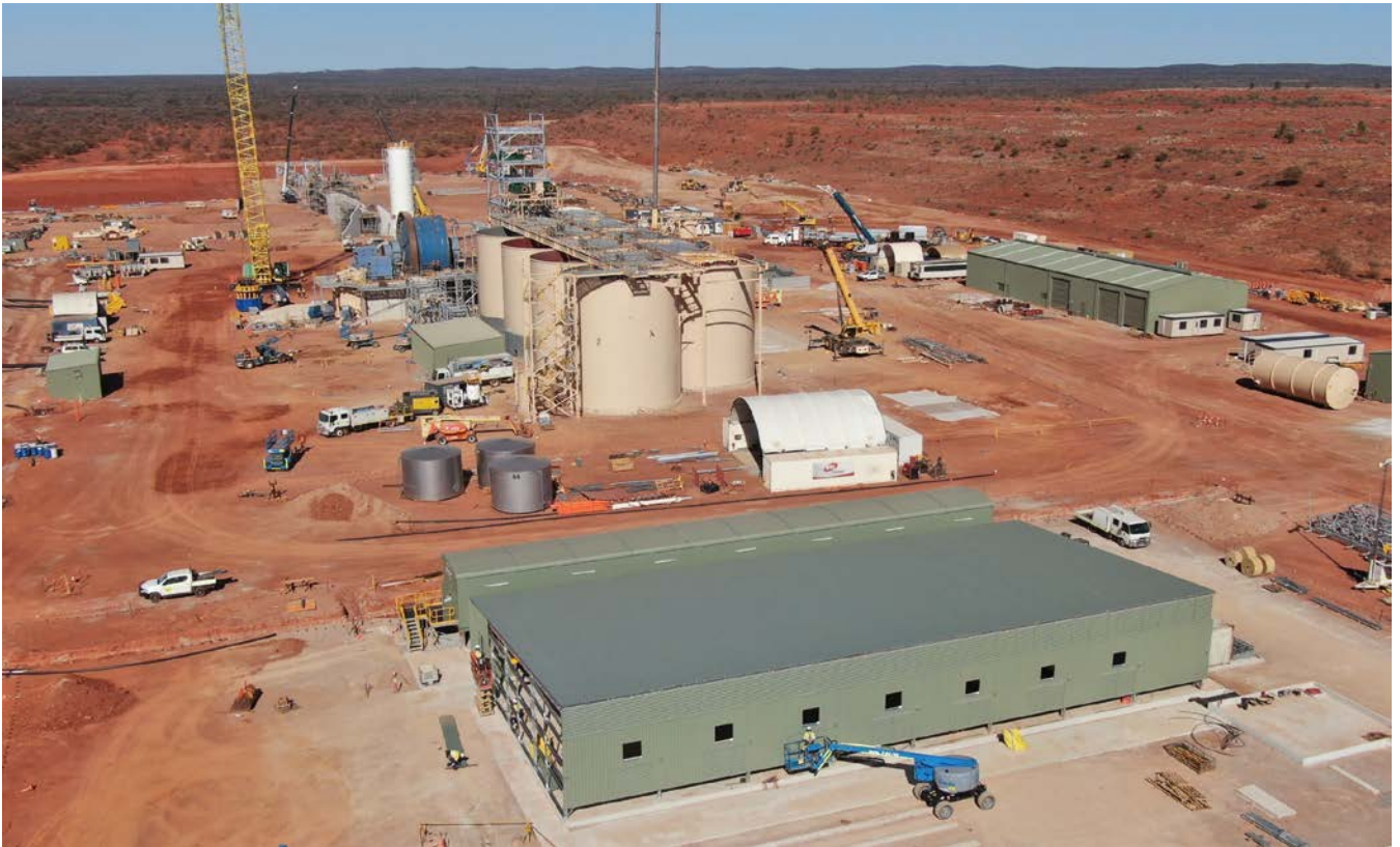
Figure 4: The power station switchroom is installed with engine hall erection nearing completion.
