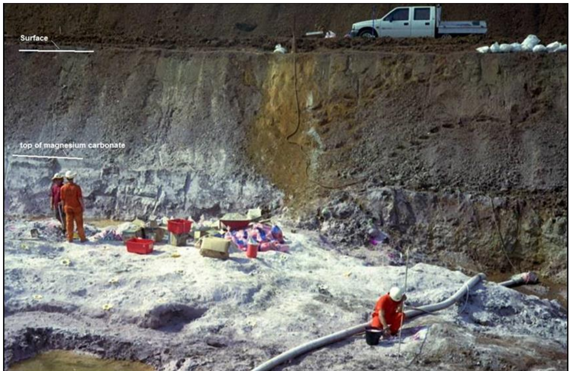
Figure 3 Test mining of magnesium at Winchester during the wet season (preparing to blast Level -1)
