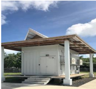
Cable Landing Stations
