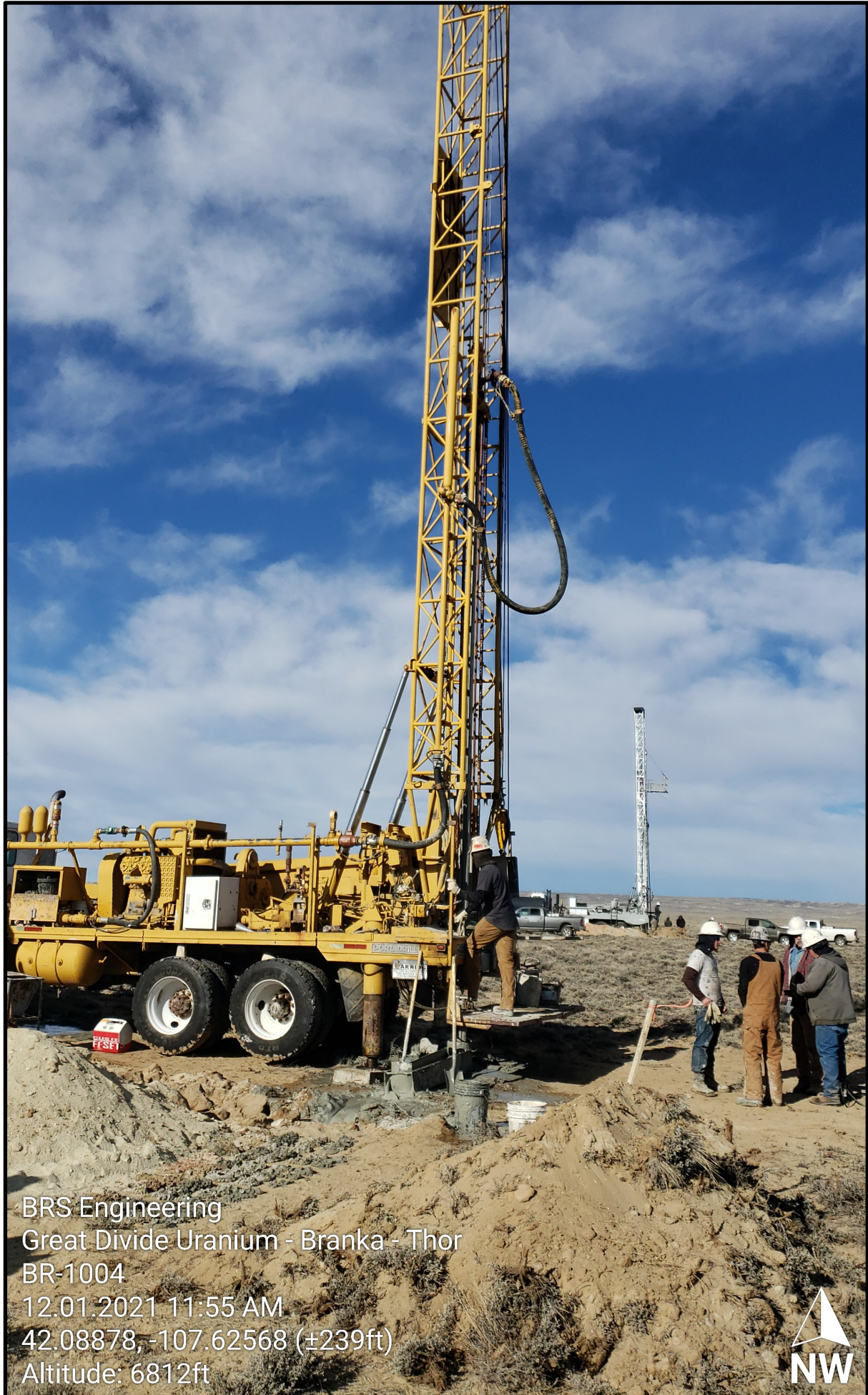
Figure 2. Mud Rotary Drill Rigs (x2), Ancillary Equipment and Support Vehicles at the Thor Project.
