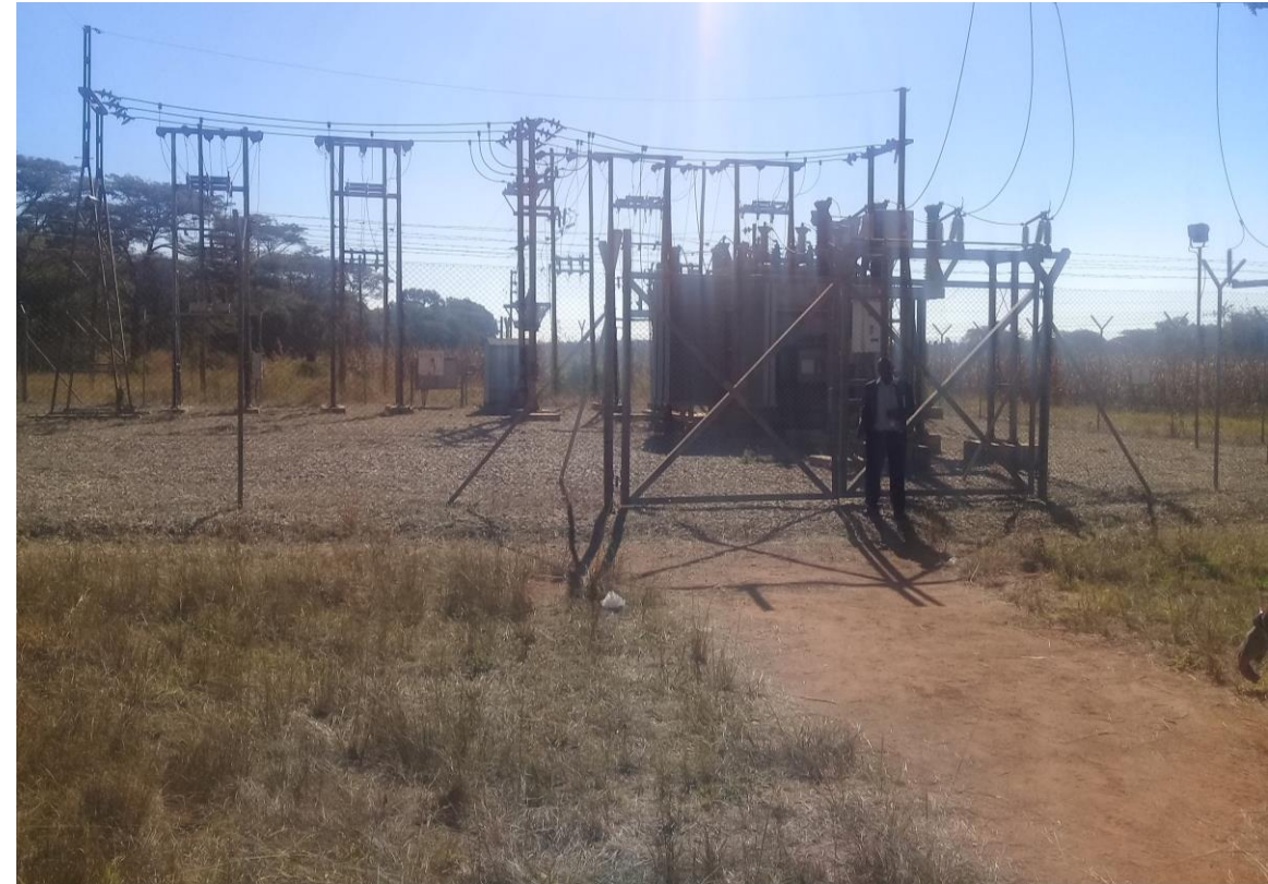
Atlanta substation located approx. 9.5km from Arcadia
