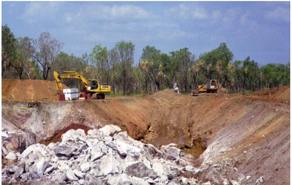
Figure 1 Test mining of magnesium at Winchester during the wet season (after blasting Level 0)
