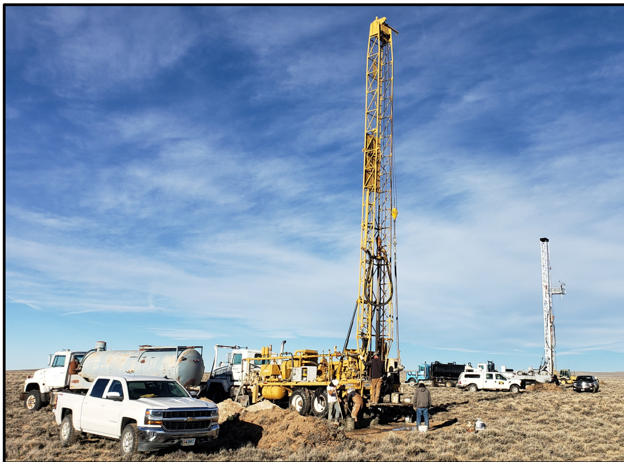
Figure 2. Mud Rotary Drill Rigs, Ancillary Equipment and Support Vehicles at the Thor Project.
