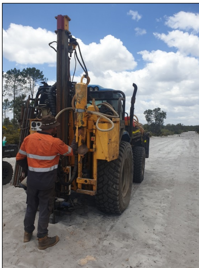
Figure 4: Vacuum drilling line 5
