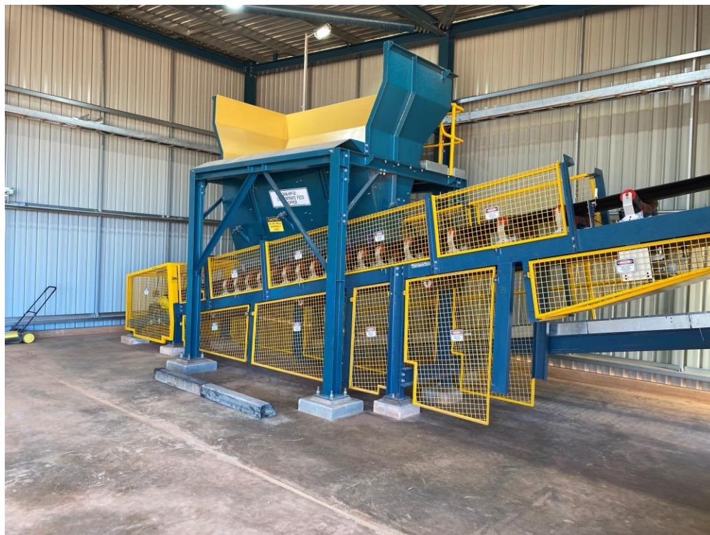
Figure 6: Packaging Feed Hopper & Conveyor
