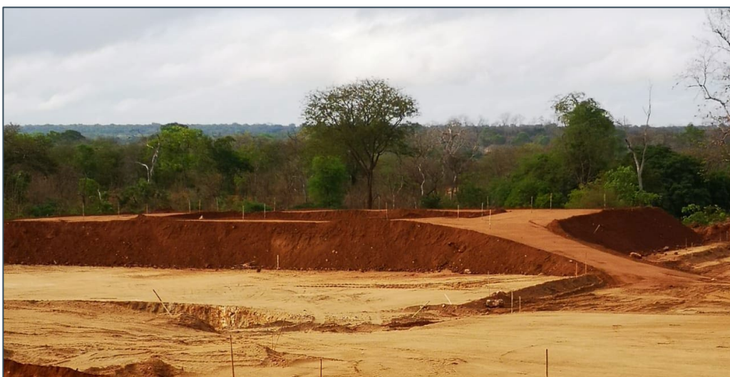
Figure 3: Raw Water Pond located within the prepared processing plant area.
