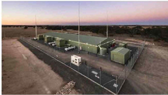
Figure 17 - ABB's Dalrymple 30MW BESS installation
