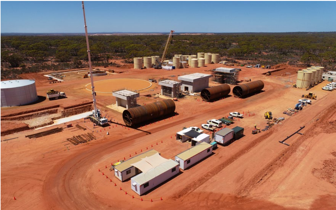
Aerial view of works completed in compliance with minor and preliminary works approval
