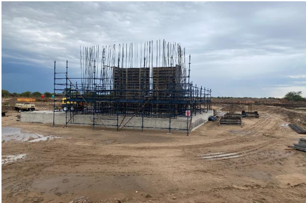
Figure 3. SAG Mill Foundation
