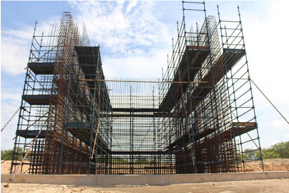
Figure 1. Primary Crusher Vault
