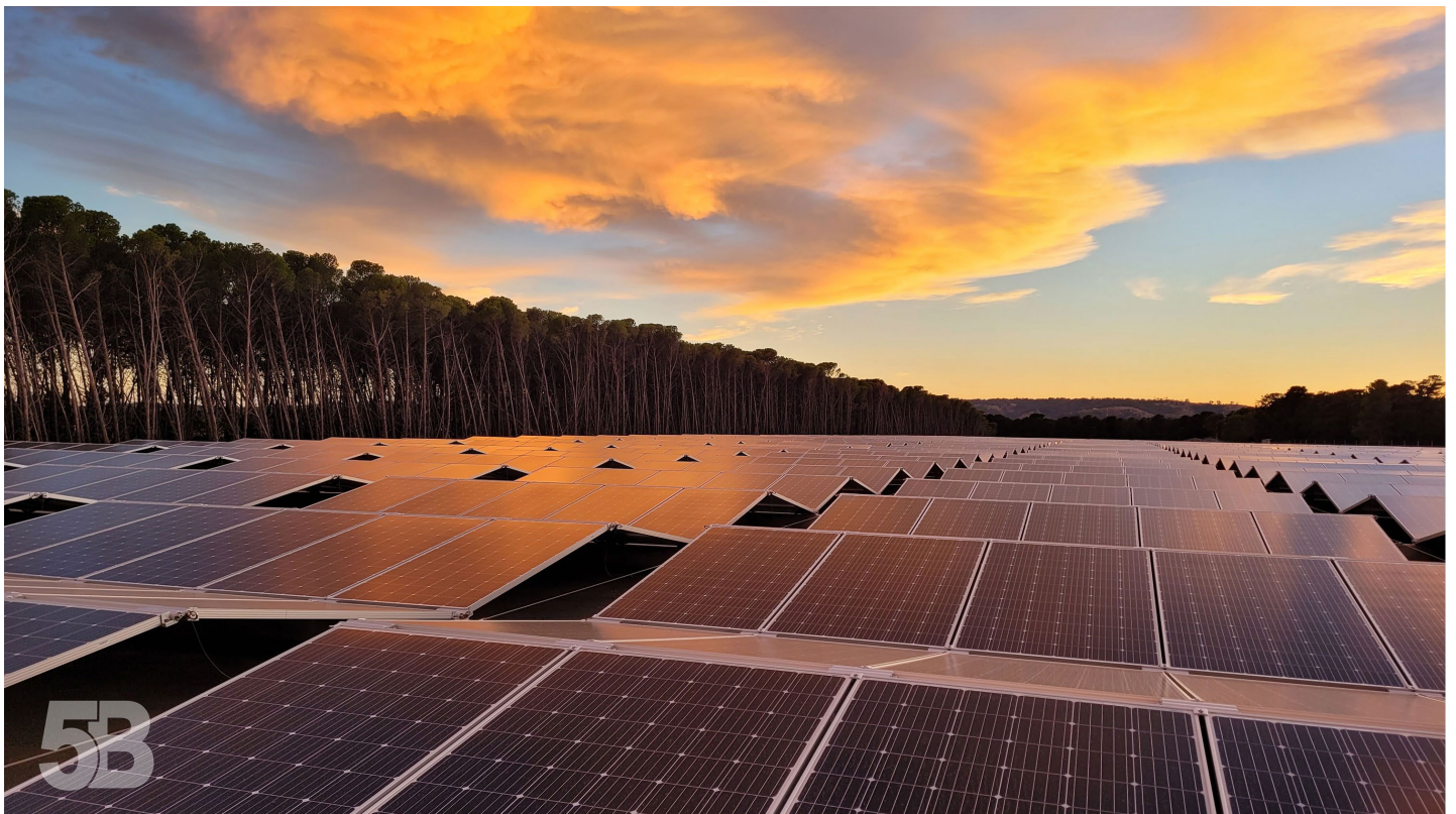
Figure 2 – Typical relocatable solar farm
