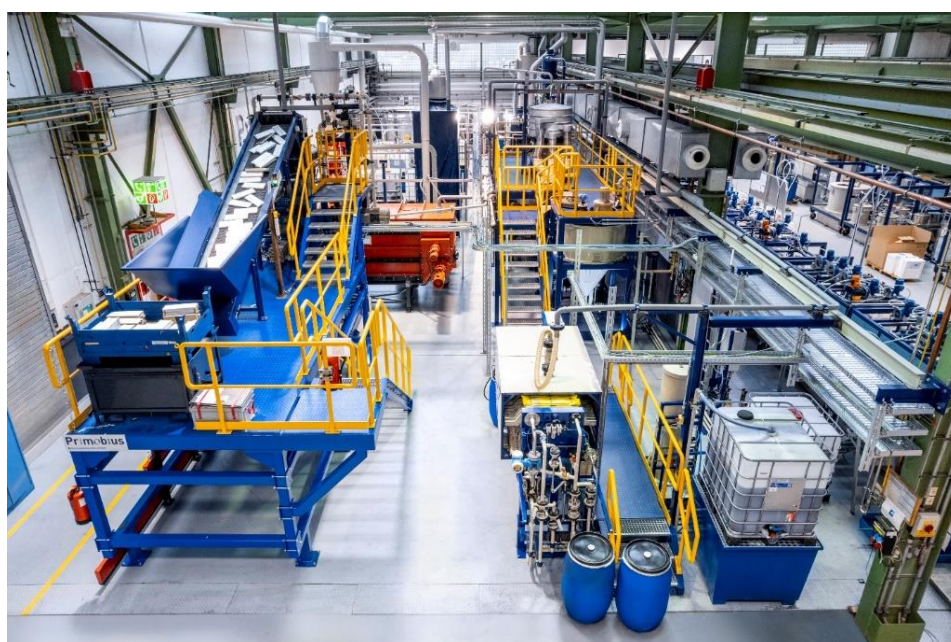
Figure 3 - Shredder and beneficiation processing EV cells
