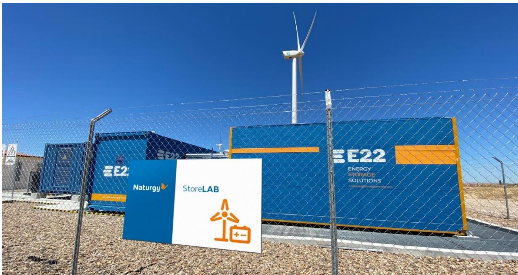
Figure 6 E22 250kW/675kWh VRFB installed in Zamora, Spain
