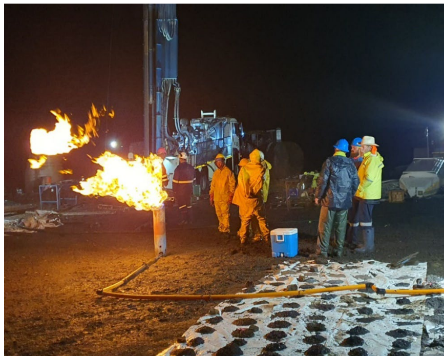
Figure 3 : Korhaan-3 Significant gas flows under downhole-choked conditions
