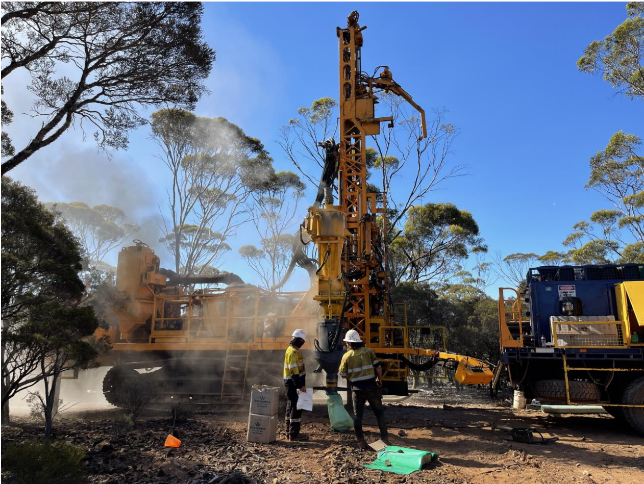
Figure 1: Drilling underway at the first drill target at Mt Deans Lithium Project
