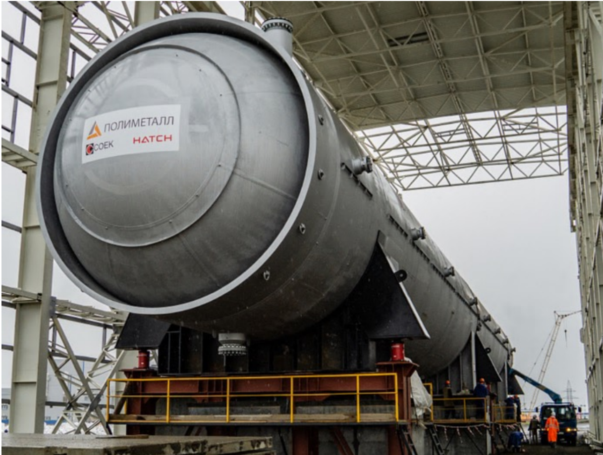
Polymetal recently installed this autoclave at their second Pressure Oxidation Plant (POX-2) in Amursk, Russia.
