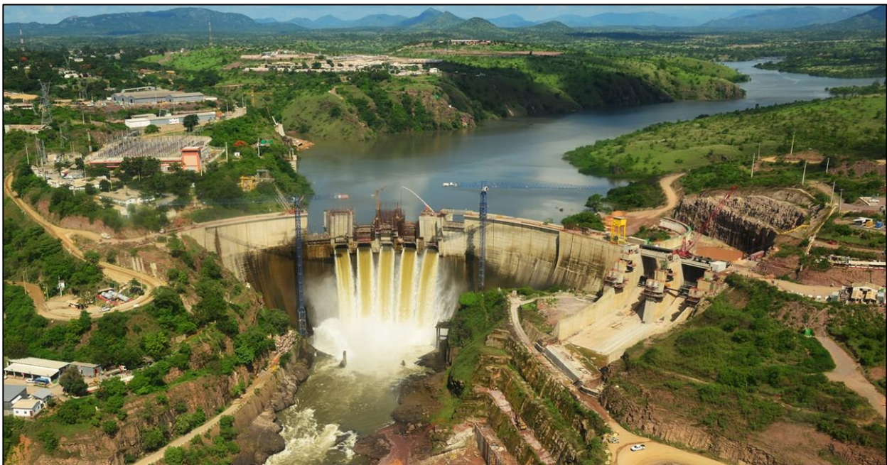
Figure 1 - Work being undertaken by Dar Al-Handasah Consultants on the Cambambe Hydroelectric Power Plant, Angola.
