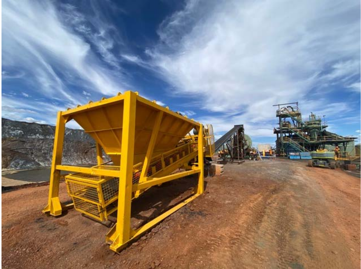
Plant front end fully commissioned
