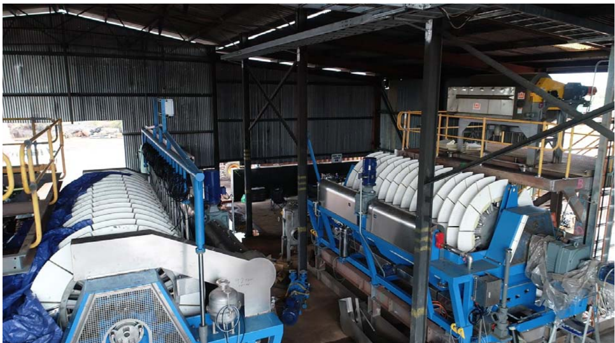
Commissioning of final stage of plant (dewatering ceramic disc filters) near completed
