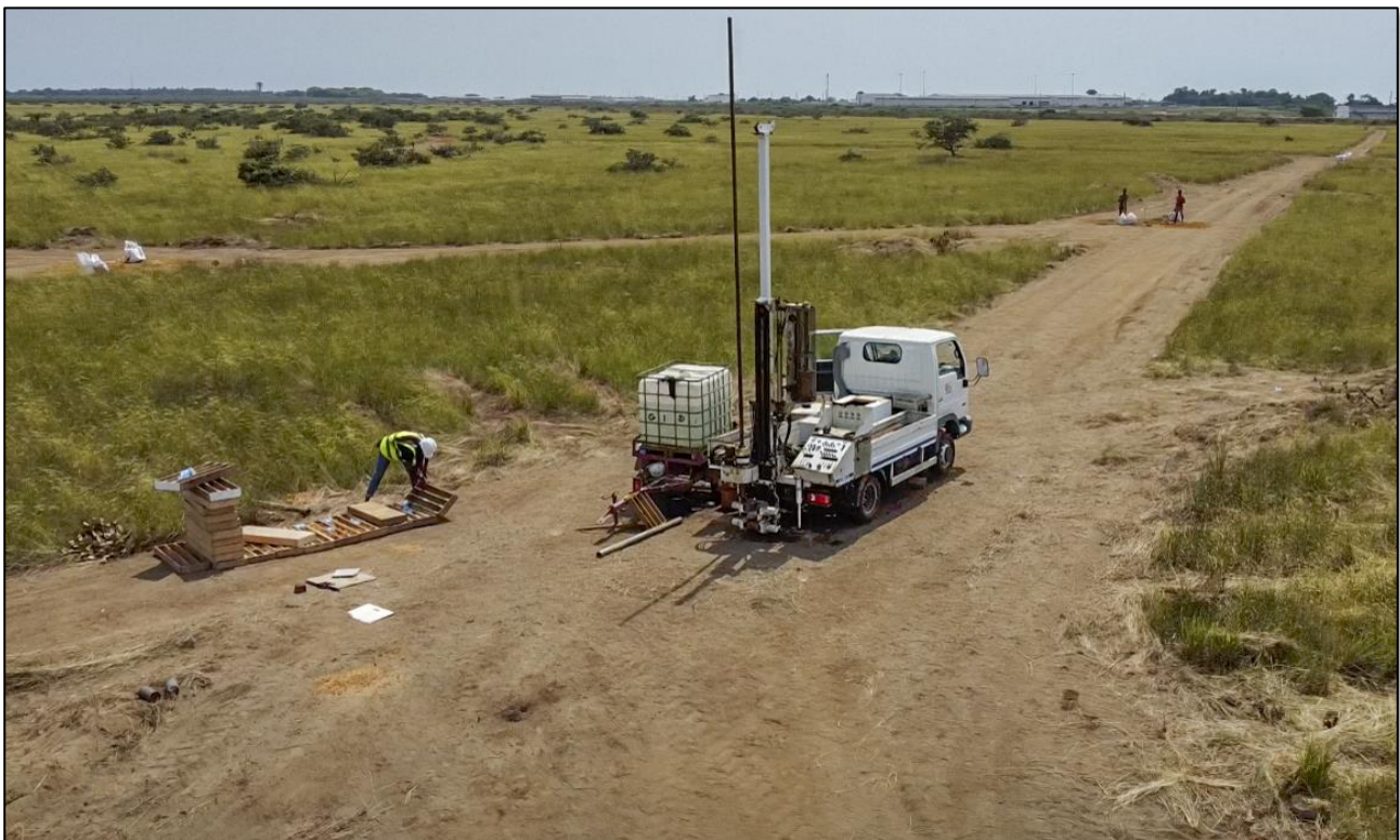
Figure 1 - Drilling works being undertaken at the site of the Cabinda Phosphate Fertilizer Plant.
