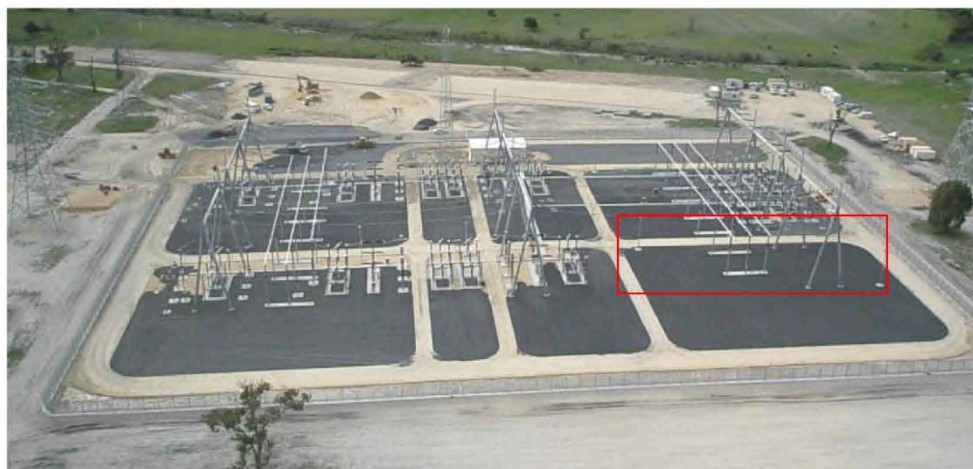
Figure 19 - LWT from south. Bay 924 can be populated to configure LWT as a secure 5-switch mesh
