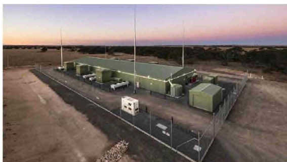
Figure 17 - ABB's Dalrymple 30MW BESS installation
