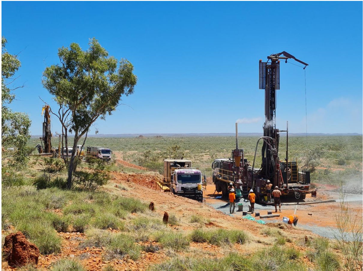
Figure 1. Photo looking west of two drill rigs currently drilling at Nil Desperandum
