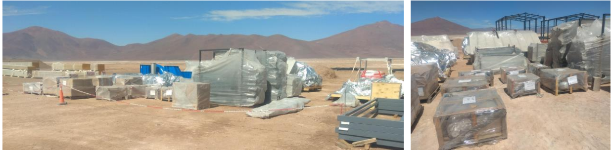
Figures 7-8. Rincon Lithium Project – 2,000tpa Operational Equipment Delivered
