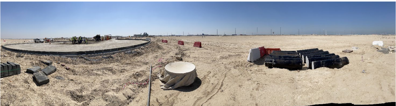
Road access, utilities and services works to the Phase 1 lot looking southwards
