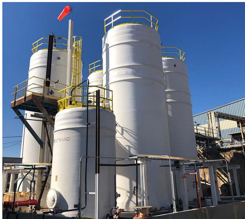
Figure 5 - USV's New VRFB Electrolyte Production Facility in Hot Springs, Arkansas.
