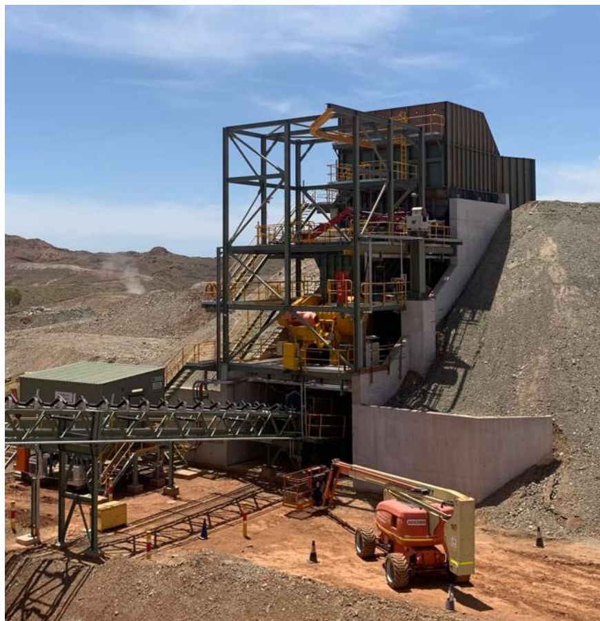
Figure 4: ROM Bin and Crusher
