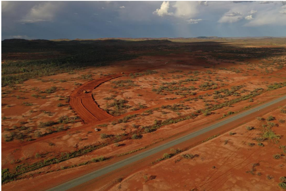
Figure 1: Commencement of Construction of Haul Road at Intersection to Public Nanutarra Road (foreground)
