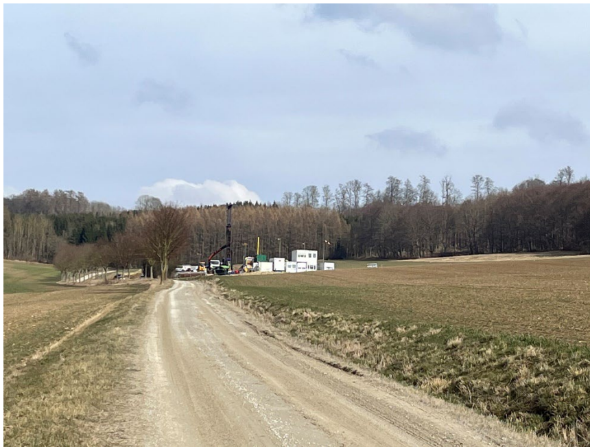
A gravel road was constructed to allow access to the drill site
