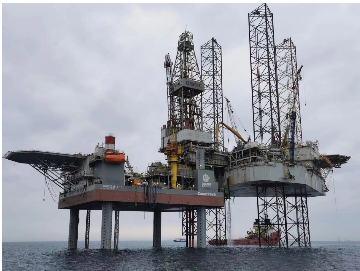
COSL Strike Rig positioned over the 12-8E platform and installing the conductors
