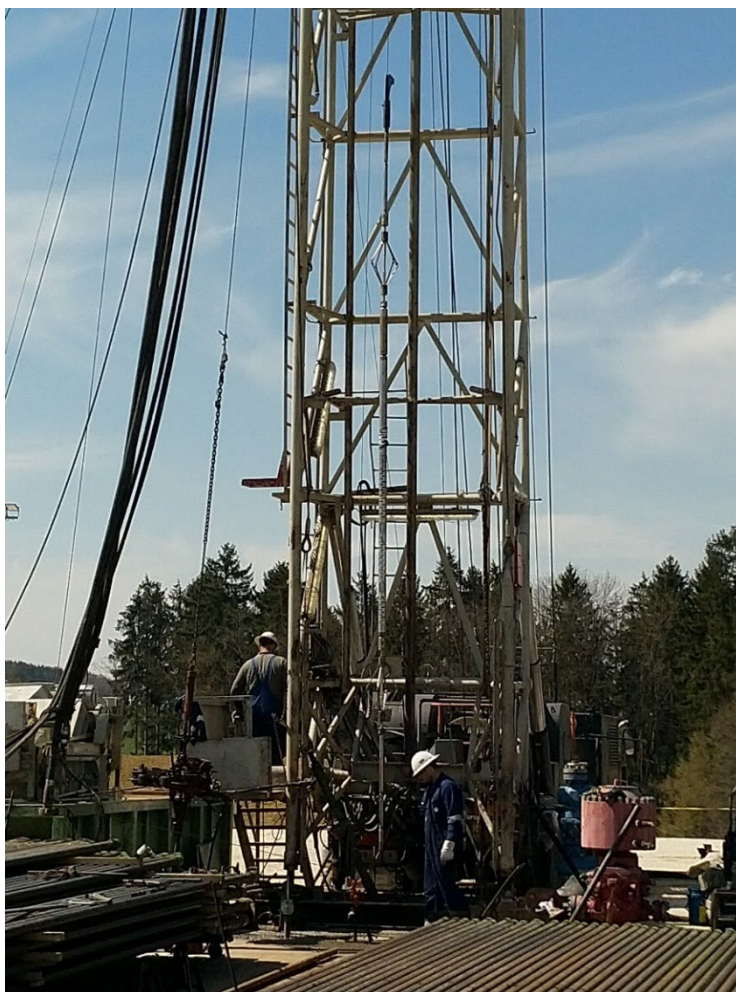
Running a cement bond survey to check well integrity of the Anshof- 3 well with the RED W-101 workover rig in preparation for testing operations. Source ADX
