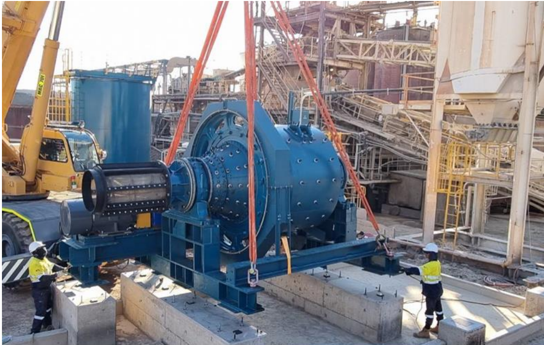
Figure 7: Refurbished Lime Slaking Mill for WilTails plan
