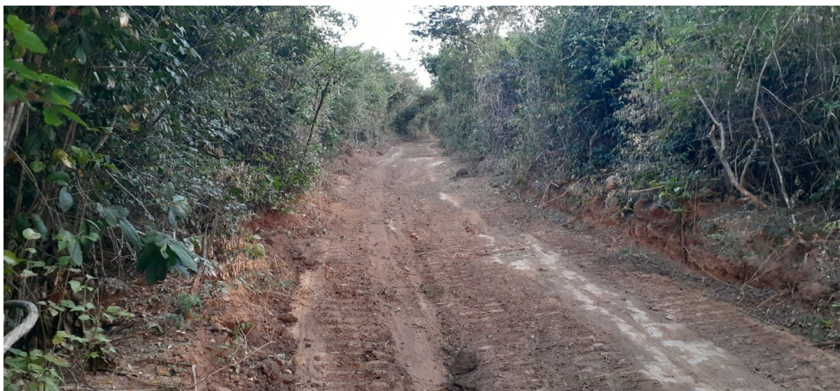
Figure 4: New site access track completed at the Monte Alto Prospect – Salinas Lithium Project, Brazil
