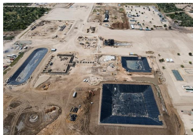
Process Plant Lined Ponds
