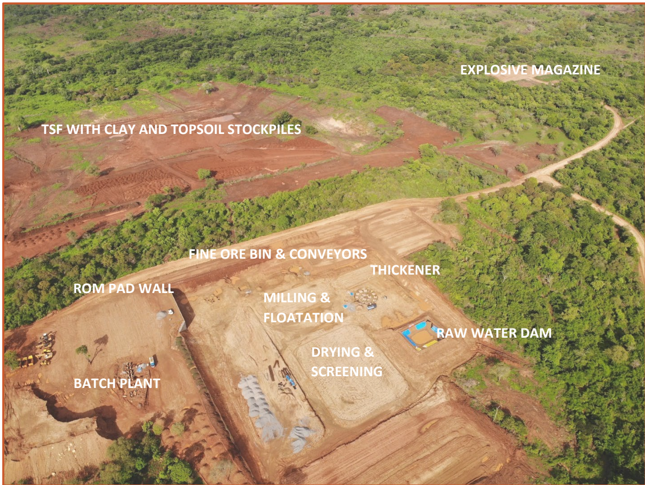
Figure 3: Aerial view (taken early February) from the southwest with the processing plant area in the foreground and the TSF in the background.
