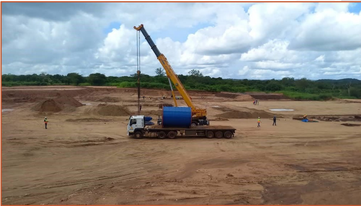
Figure 1: Offloading of the rod-mill on site using the Lindi Jumbo 55 tonne mobile crane.
