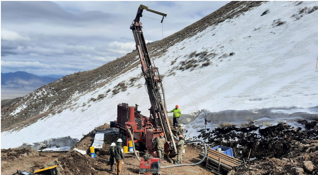
Figure 10 RC percussion drill rig on site drilling the first hole at Star Canyon, Nevada
