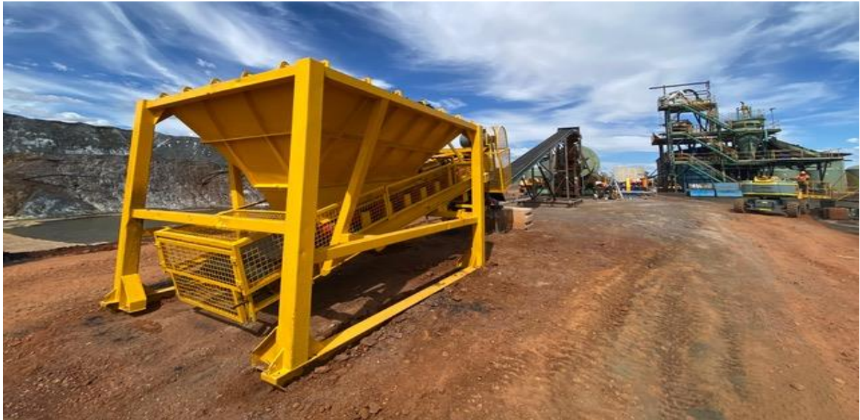
Plant front end fully commissioned
