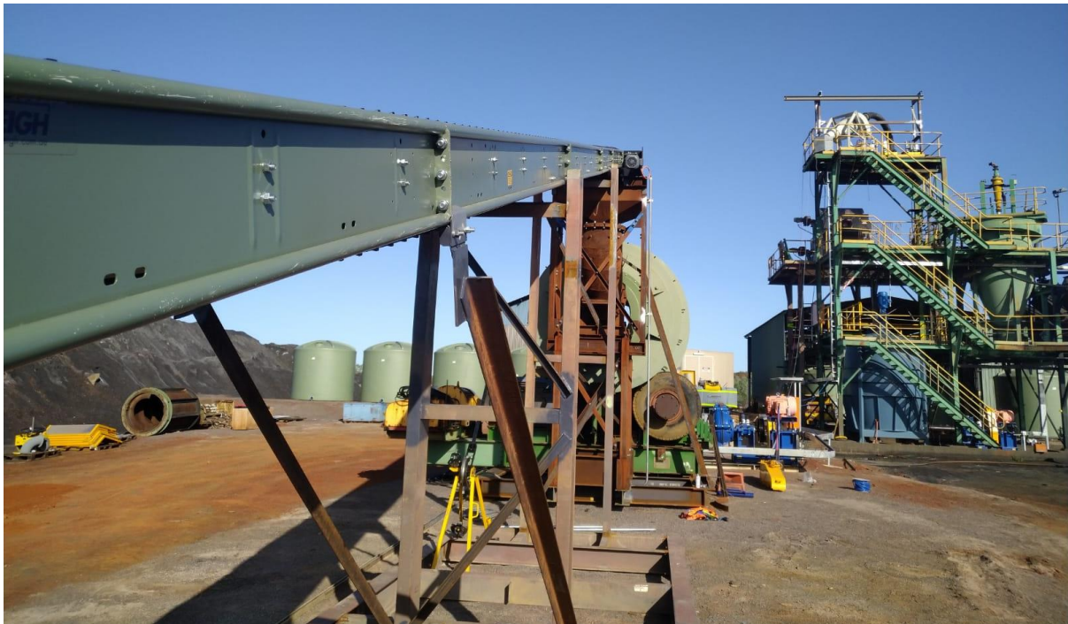
Process water tanks, mixing tanks, cyclone and magnetic separator tower in the background
