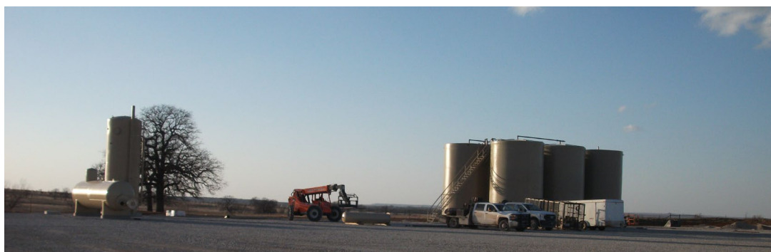
Figure 4. Rangers tank battery and separators
