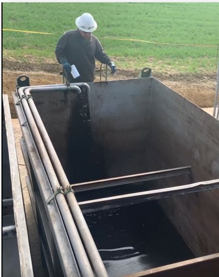
Photograph of Anshof-3 Production Test
